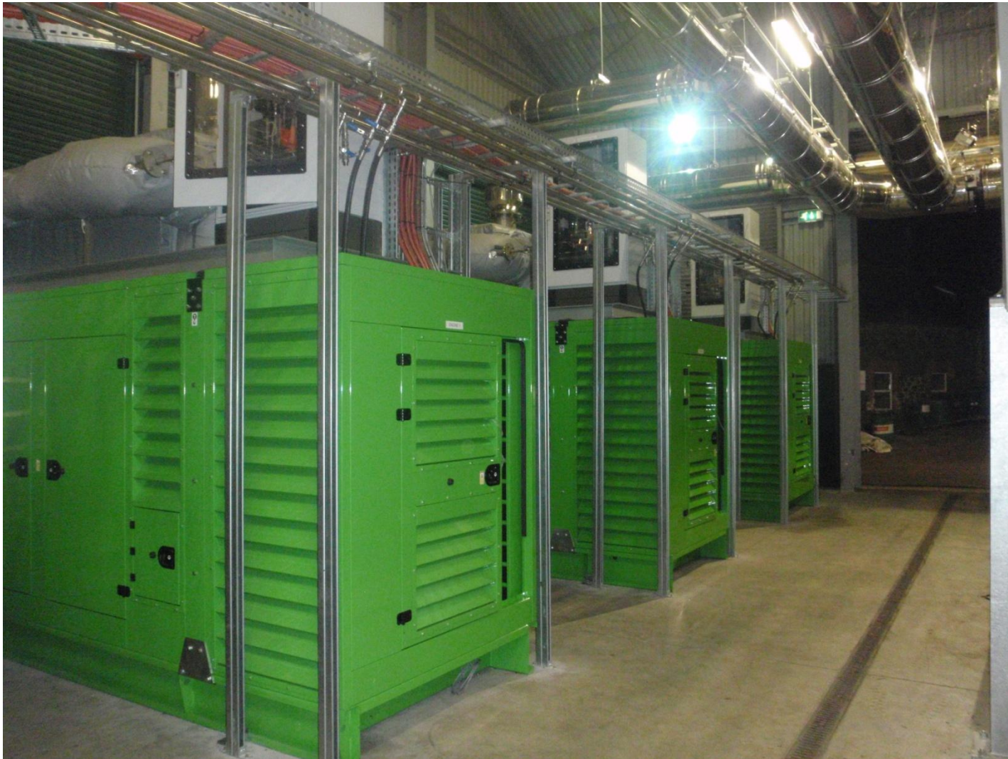
Aquafuel 1.5 MW CHP installation in a tallow plant in Northern Ireland
